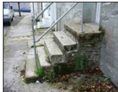
Granite steps to raised front doors are a local detail in the Fore Street area
