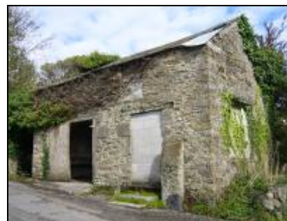
A number of outbuildings survive but are vulnerable to loss
